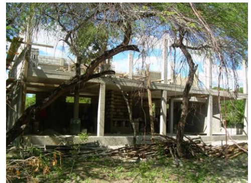
CENEOH (Center for Neohumanist Education) under construction. The planned center will be powered by a solar PV panel system, and will house a conference hall, offices, a teacher resource library, a computer and fast speed Internet space, and a yoga studio.
